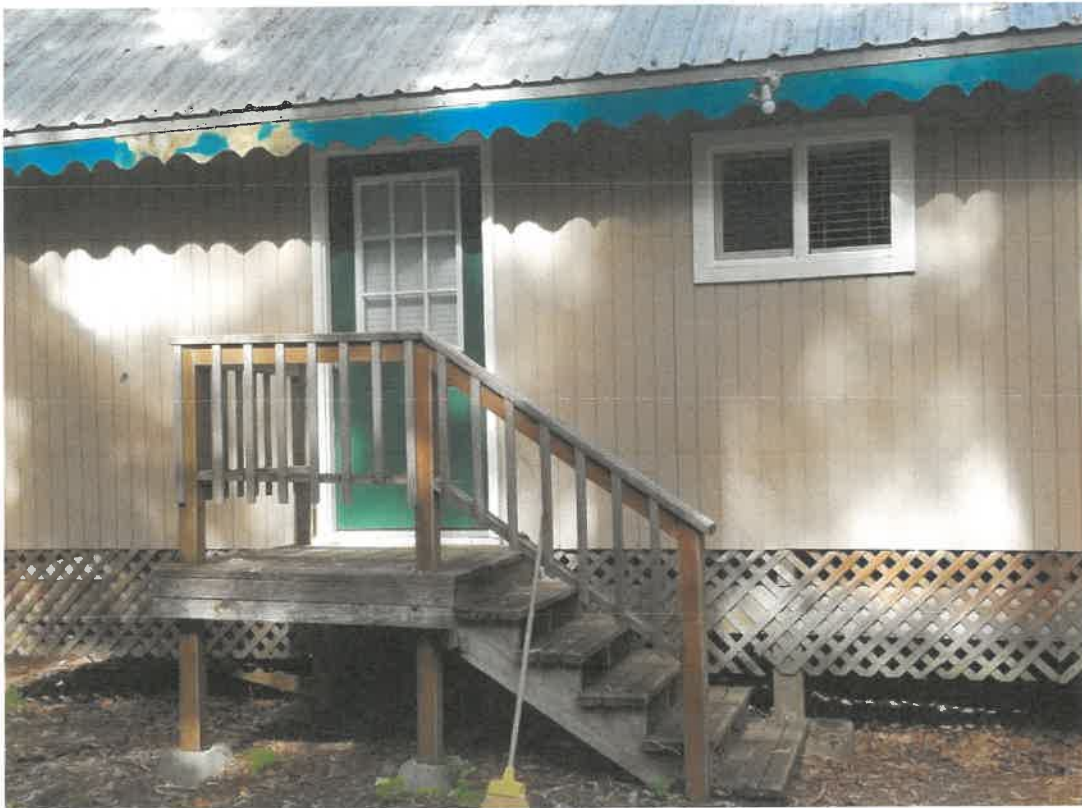
Front porch still standing but to be replaced.
